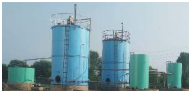
Fig 1: AD pilot scale (50 M3) digesters at Nira-Bhima SSK
